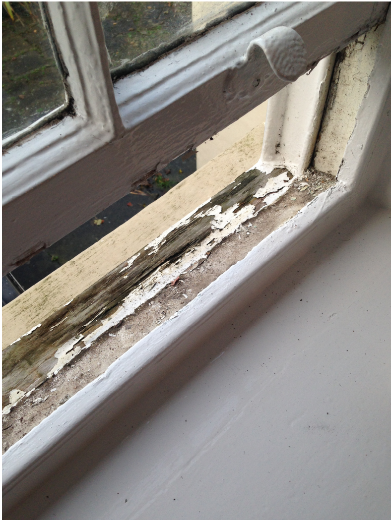
Fig.2 – Example of rotten existing windows requiring replacement.
