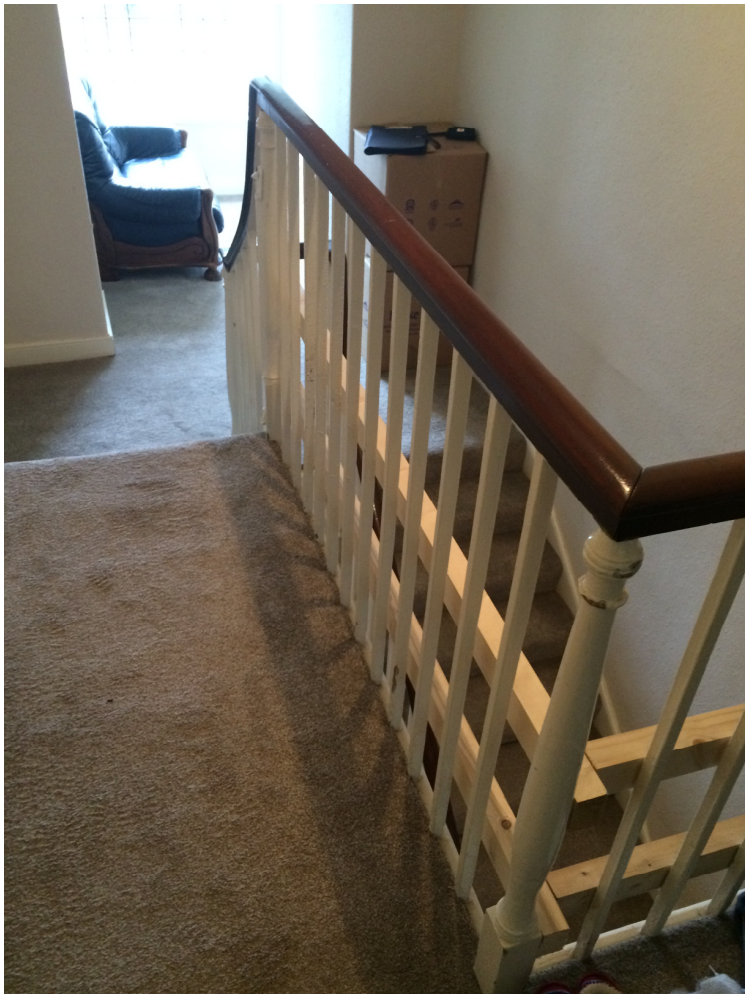
Fig.5 - View of existing staircase to be replaced indicating temporary timber safety rails.
